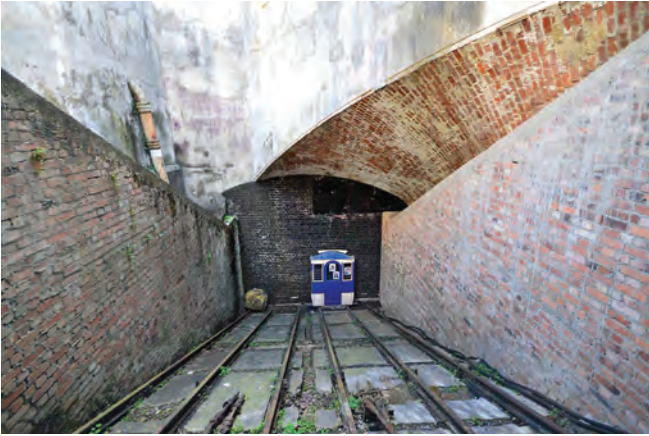
Top of the Rocks Railway with two full pairs of tracks in the centre (one has a model railway car at its base), and single rails only of the two outer tracks (the other rails would have run where the stairs were installed behind the wartime blast walls)
